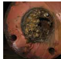
▲ Cross-section view of water pipe blocked by mussels.
